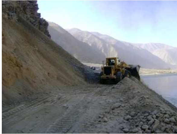
An excavation of the road from Kishim to Fayzabad as part of a U.S. Agency for International Development project. Photo by: USAID Afghanistan / CC BY-SA
