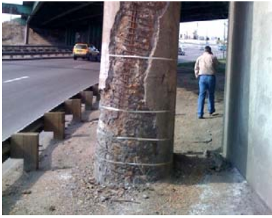
crumbling bridge support in Colorado. (Photo: Pure Thinking )
